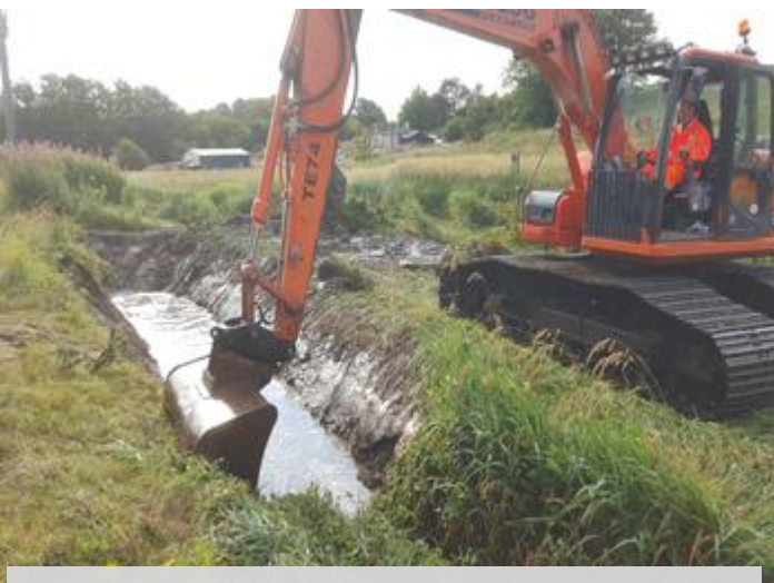
Excavated material was deposited on the lineside, graded and compacted to leave a level safe site.
