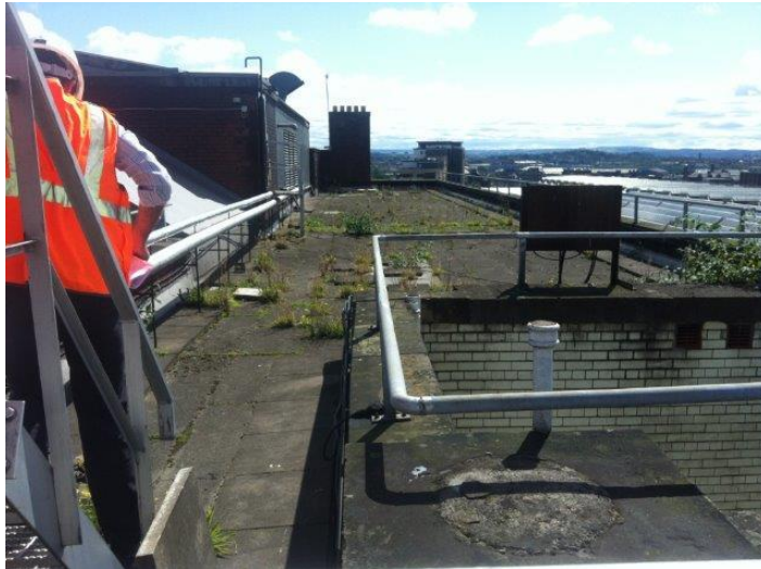
Rear of the roof before we started, and below showing new roof membrane, pipe supports and fascia to high roof level.
