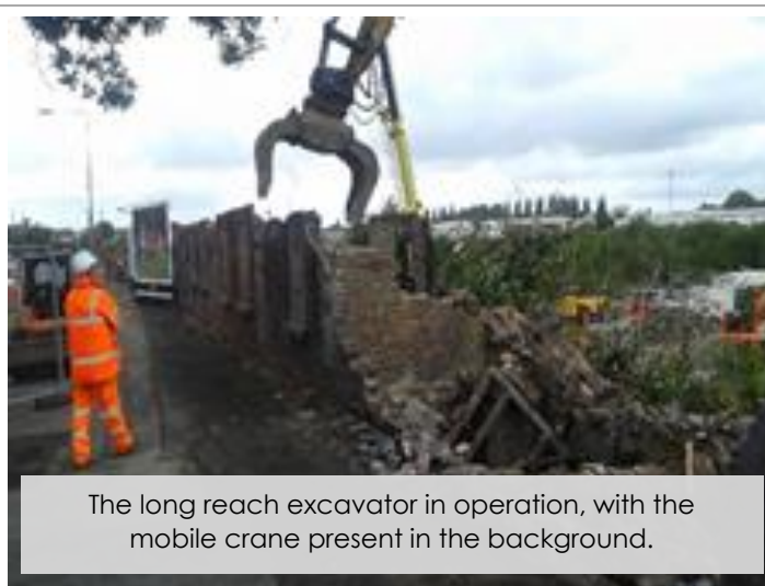
The building was quickly deemed to be dangerous and required immediate removal.
