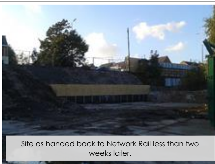
The long reach excavator in operation, with the mobile crane present in the background.
